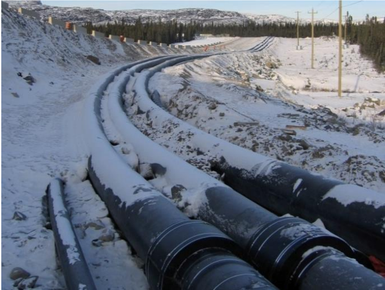
Freeze control pipes
